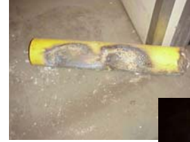
Items cut during Demolition causing soot
